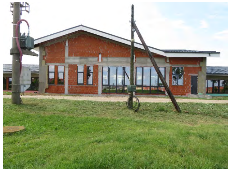
Above: The new accommodation block for adults with disabilities is progressing well.
