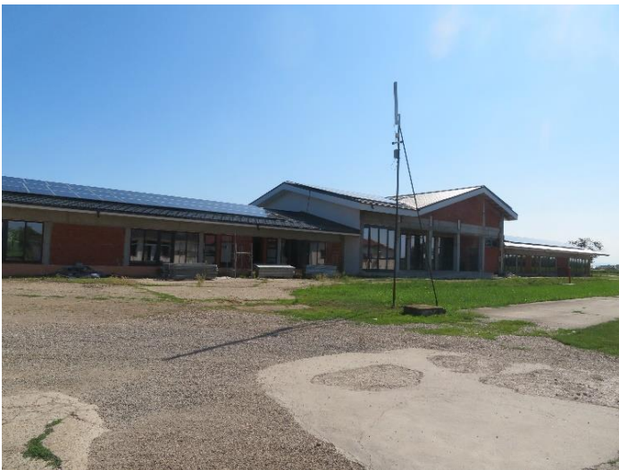
Above: Progress is good in the completion of the new accommodation block.
